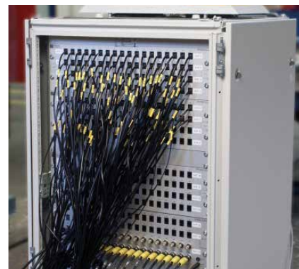
Data Acquisition System (288 channels)
